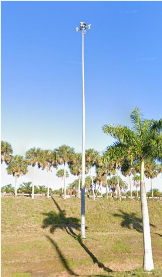
High Mast Light Pole
